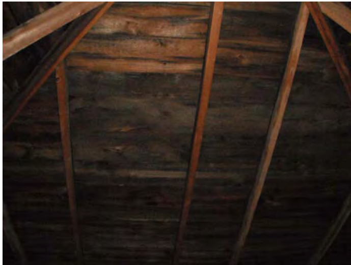
Inadequate and randomly spaced rafters
