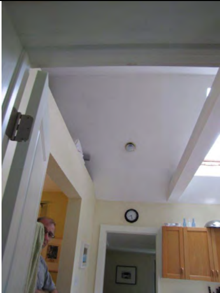
Most of the cathedral ceiling in the kitchen shows some heat loss.
