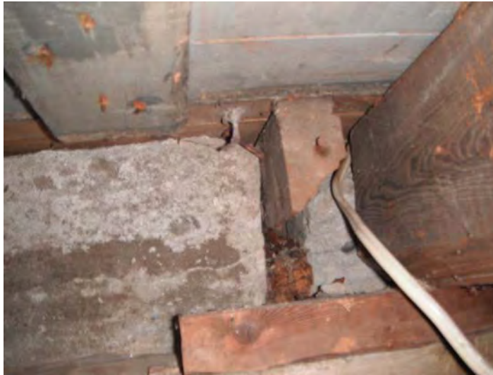
Concrete infill and rotted joist
