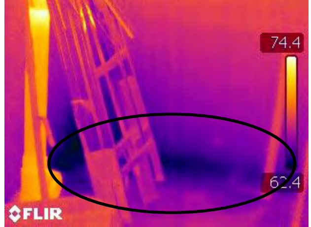
Moisture intrusion occurring at floor height.
