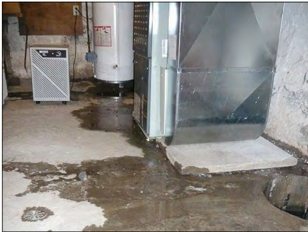
Groundwater seepage in the basement.
