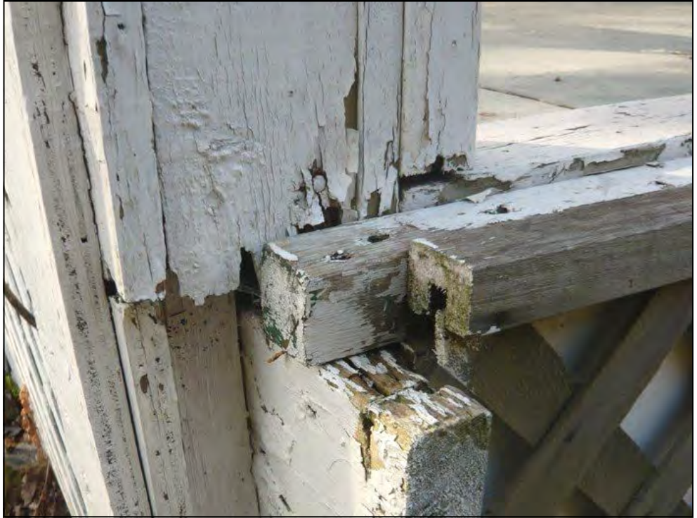
Poor condition of the porch.
