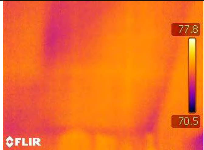
The heat loss may affect the roof in winter months causing ice damming because of insufficient ventilation.
