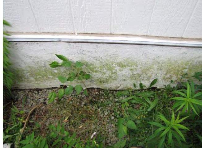
No access available to the crawlspace under the bathroom at the side of the home or the crawlspace at the front of the home.
