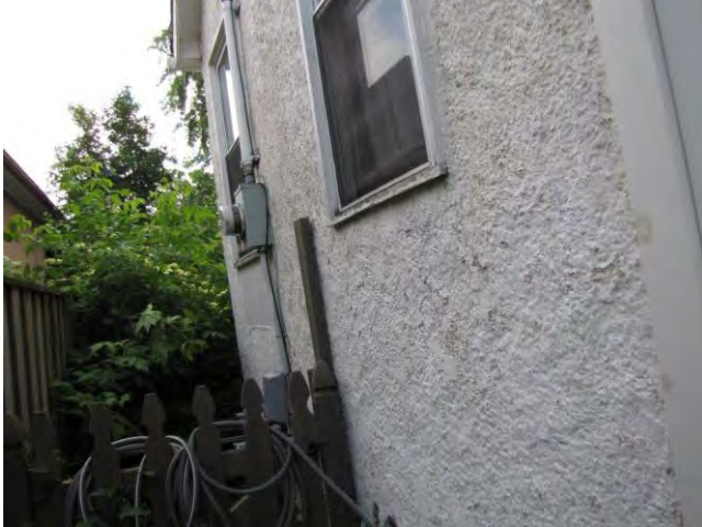
Wood trim is built into the stucco finish. The trim is deteriorating around windows.
