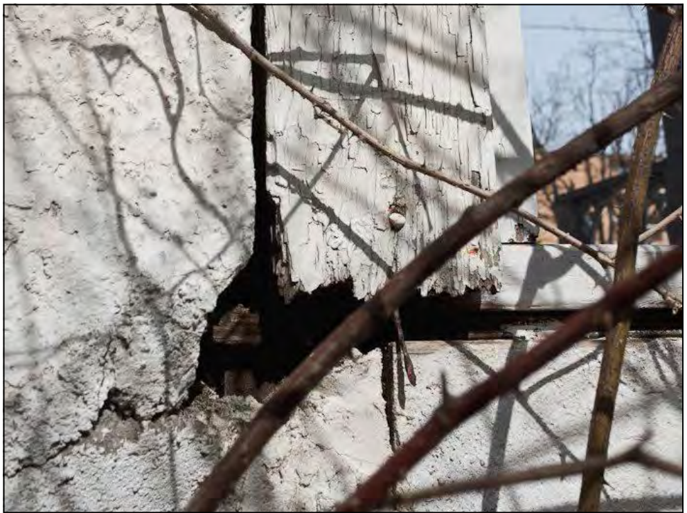
Rotting wood and chipped stucco.
