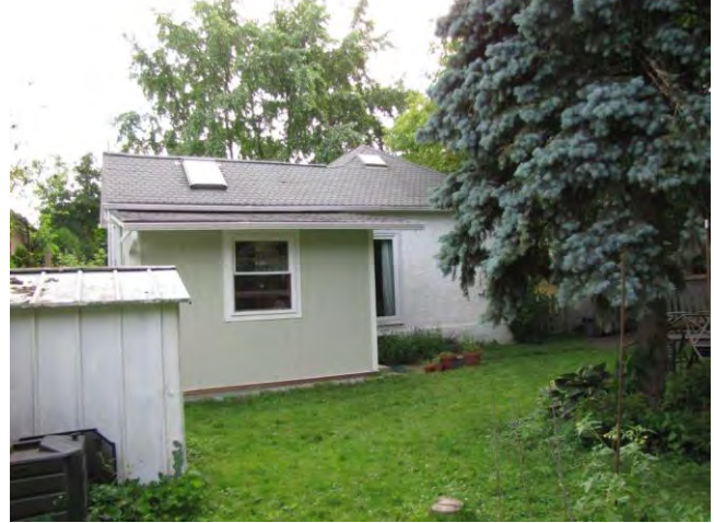
Unvented attic over addition, unvented main attic and unvented cathedral ceiling cavities. All roof/attic spaces are prone to condensation and mold growth because of insufficient ventilation.
