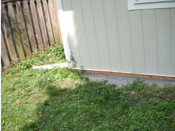
Rear addition with improper foundation and moisture protection
