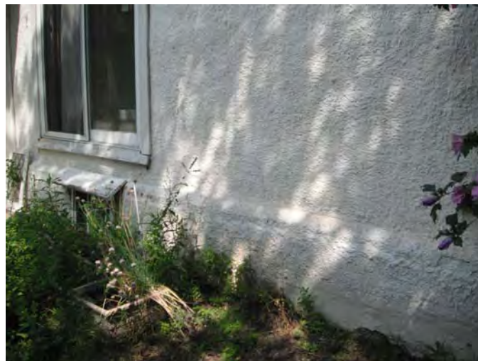
Misaligned foundation at rear wall
