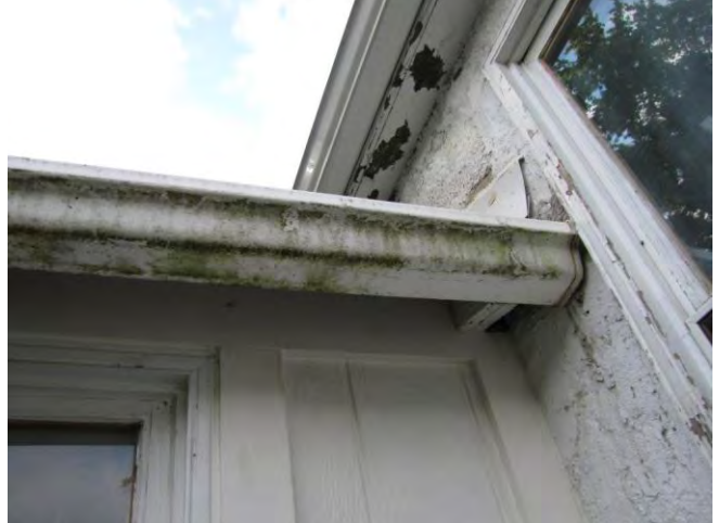
Photo 10: Poor drainage at Eavestrough
