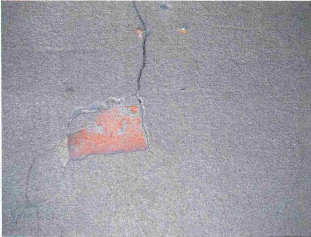
Photo 6, Spalled Interior Brick
