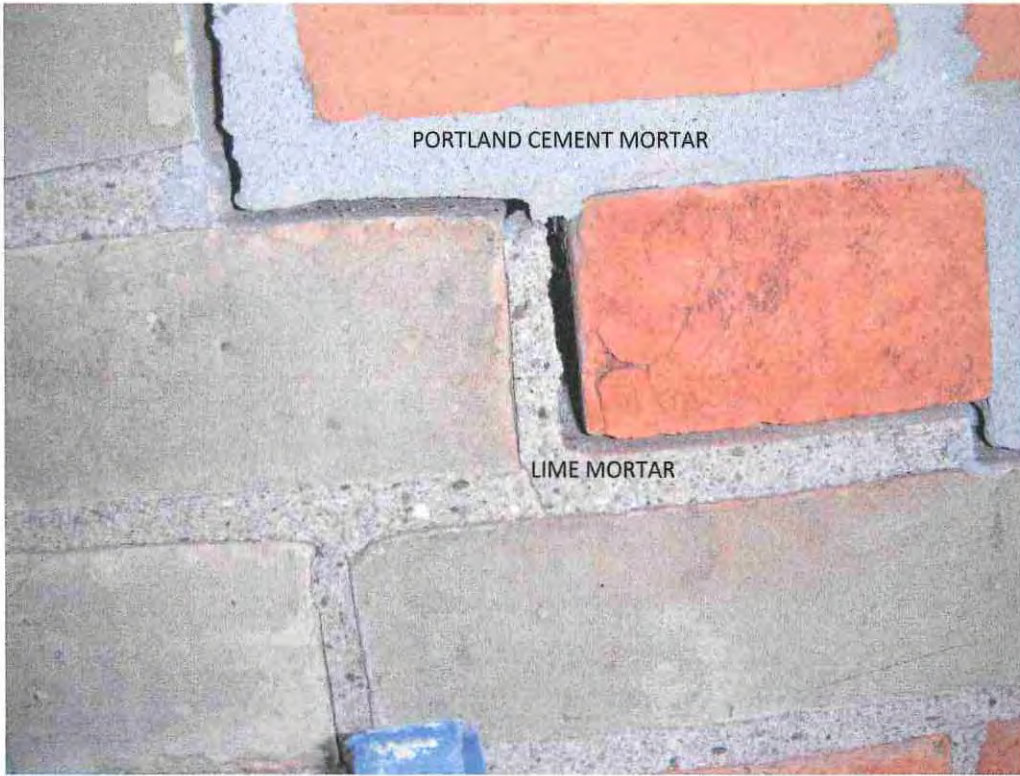
Photo 5, Inappropriate Repair Material
