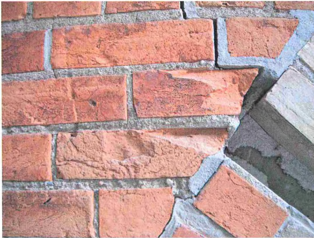
Photo 4, Damaged Brick Faces
