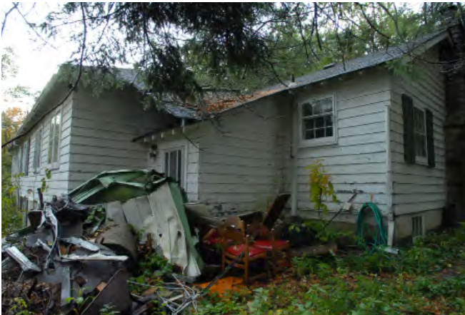
North East Corner (Note awkward roof condition at Rear Entry)
