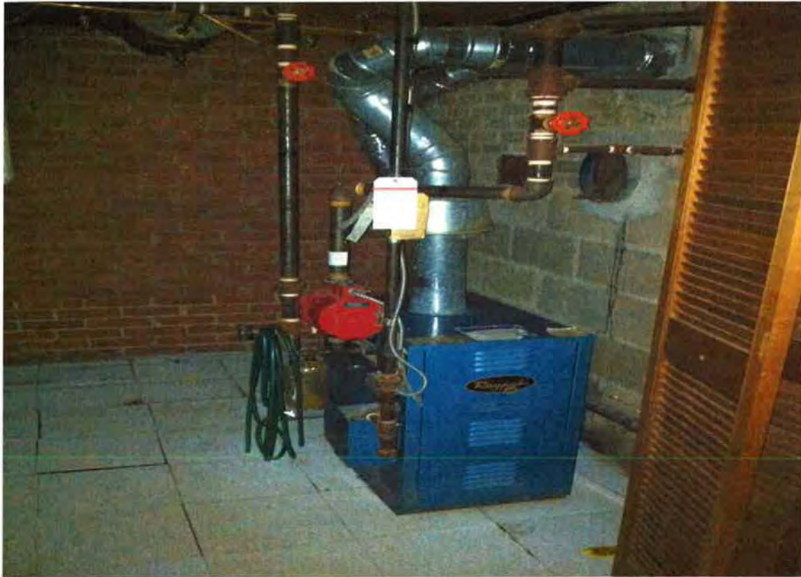
EXISTING FURNACE SYSTEMS
