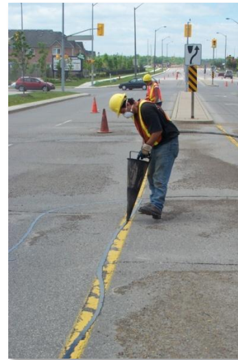
Crack filling/sealing prevents water from entering the road base and is a cost effective way to maintain the pavement assets
