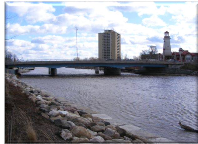
The Credit River bridge on Lakeshore Road Originally built in 1960 and rehabilitated in 2007
