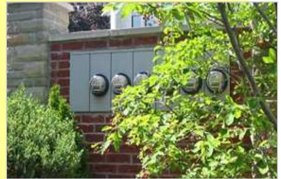
Decorative wall to conceal hydro meters
