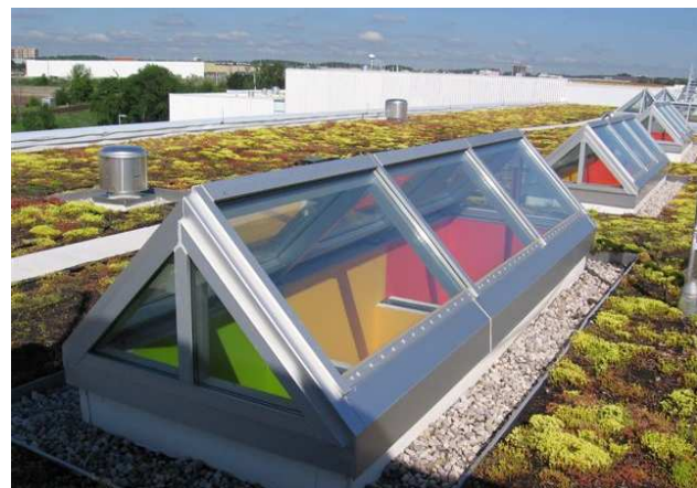
Figure 9-38: Green roofs are an effective stormwater best management practice and contribute to the reduction of the urban heat island effect.
