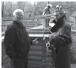
Fred Durdan and John Van Camp of the Log Cabin Task Force give a "thumbs up" to the construction underway for the Log Cabin basement.
