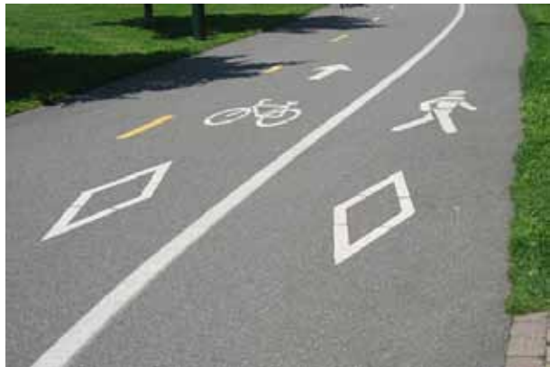
Figure V-15: Example of separated path in Quebec City, which runs both in street boulevards, and on its own alignment along the waterfront.
