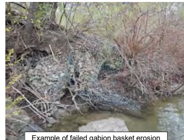
Example of failed gabion basket erosion control protection within the Study Area.
