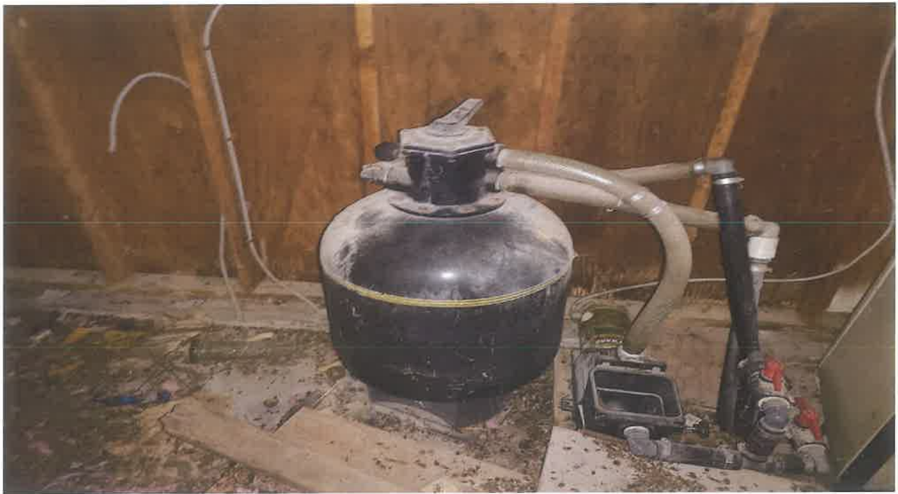
Pool Filter System within Garage on subject site (looking south)
