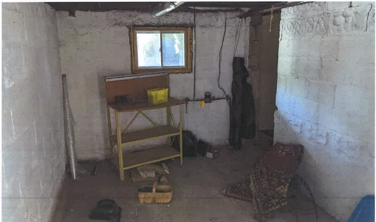
View of household garbage in the basement of the residential building at 1022 Caven Street
