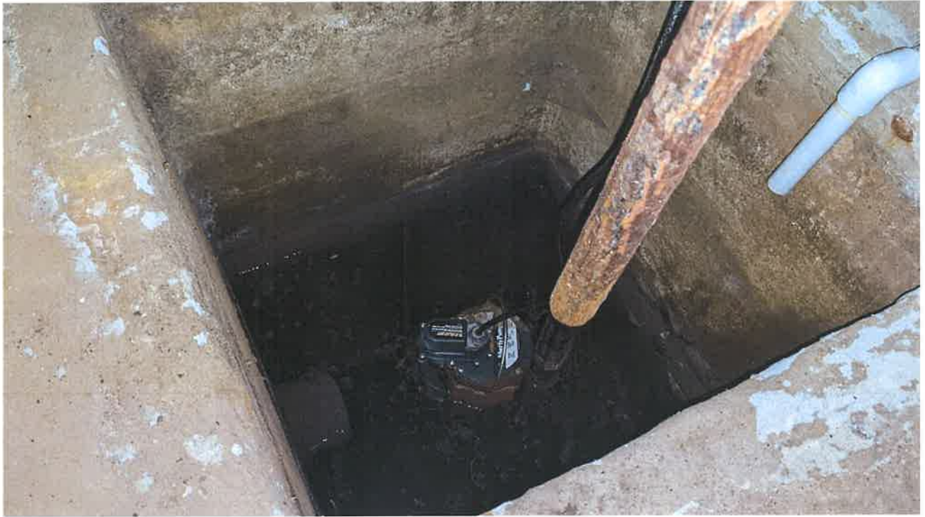
View of sump pump located at basement of 585 Lakeshore Road East
