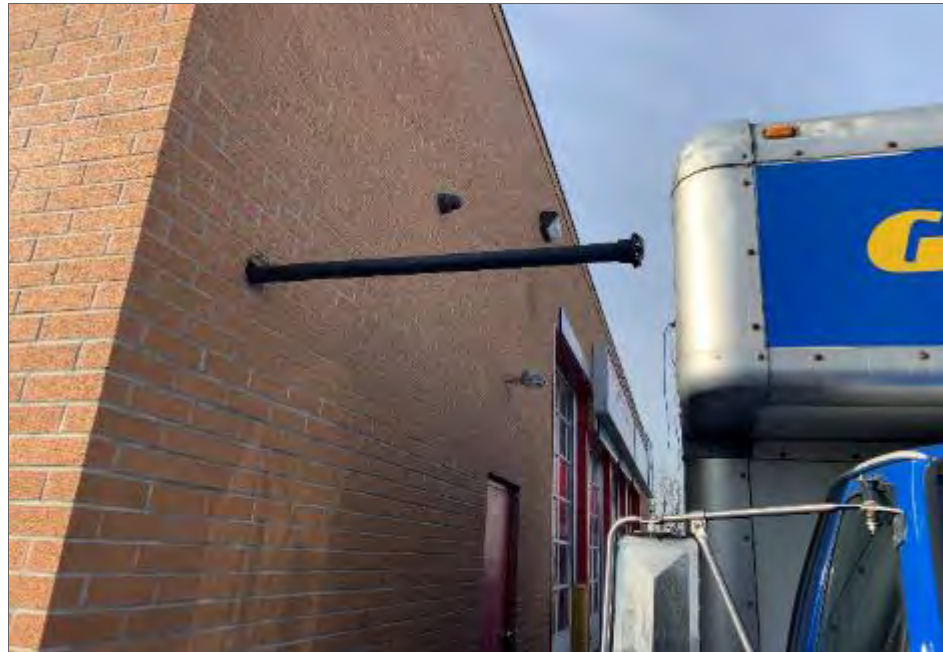
Photo 10 – Vent pipe located on the north exterior portion of Site Building A, facing southwest.
