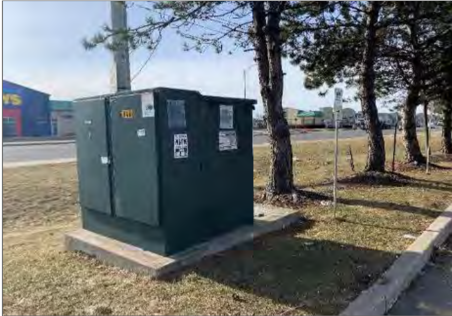
Photo 21 – Transformer located in the east portion of the Site, looking southwest
