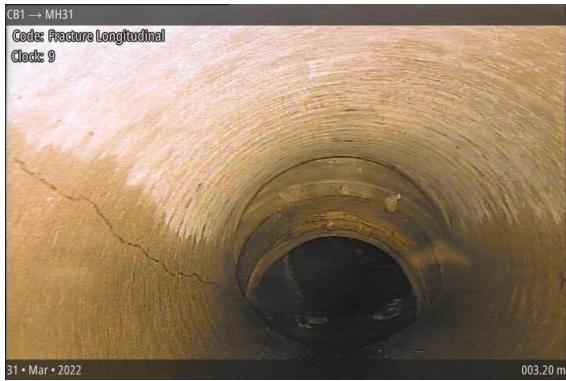
Fracture Longitudinal at 003.20 m, 9 o'clock
