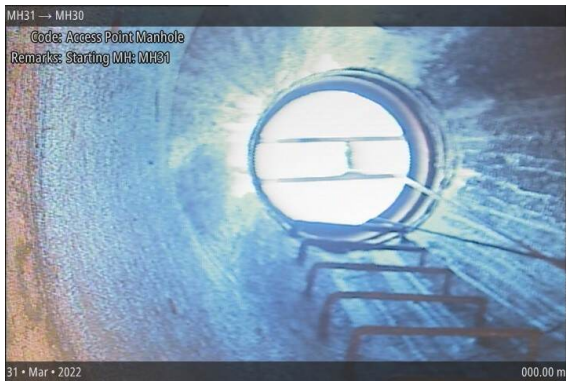
Access Point Manhole at 000.00 m | Starting MH: MH31
