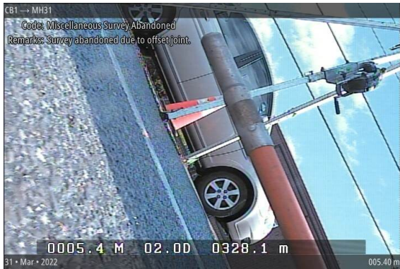
Miscellaneous Survey Abandoned at 005.40 m | Survey abandoned due to offset joint.
