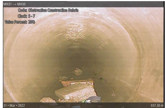
Obstruction Construction Debris at 037.30 m, 5 - 7 o'clock
