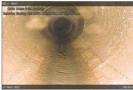
Access Point Manhole at 000.00 m | Starting MH: MH31. Cannot view MH due to slope.
