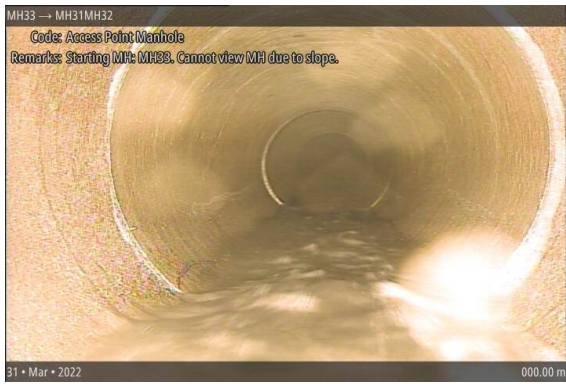
Access Point Manhole at 000.00 m | Starting MH: MH33. Cannot view MH due to slope.
