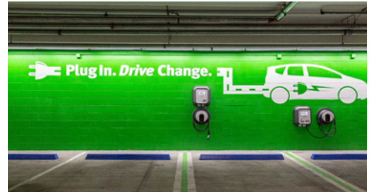
Figure 20: Example of an Electric Plug-in Station
