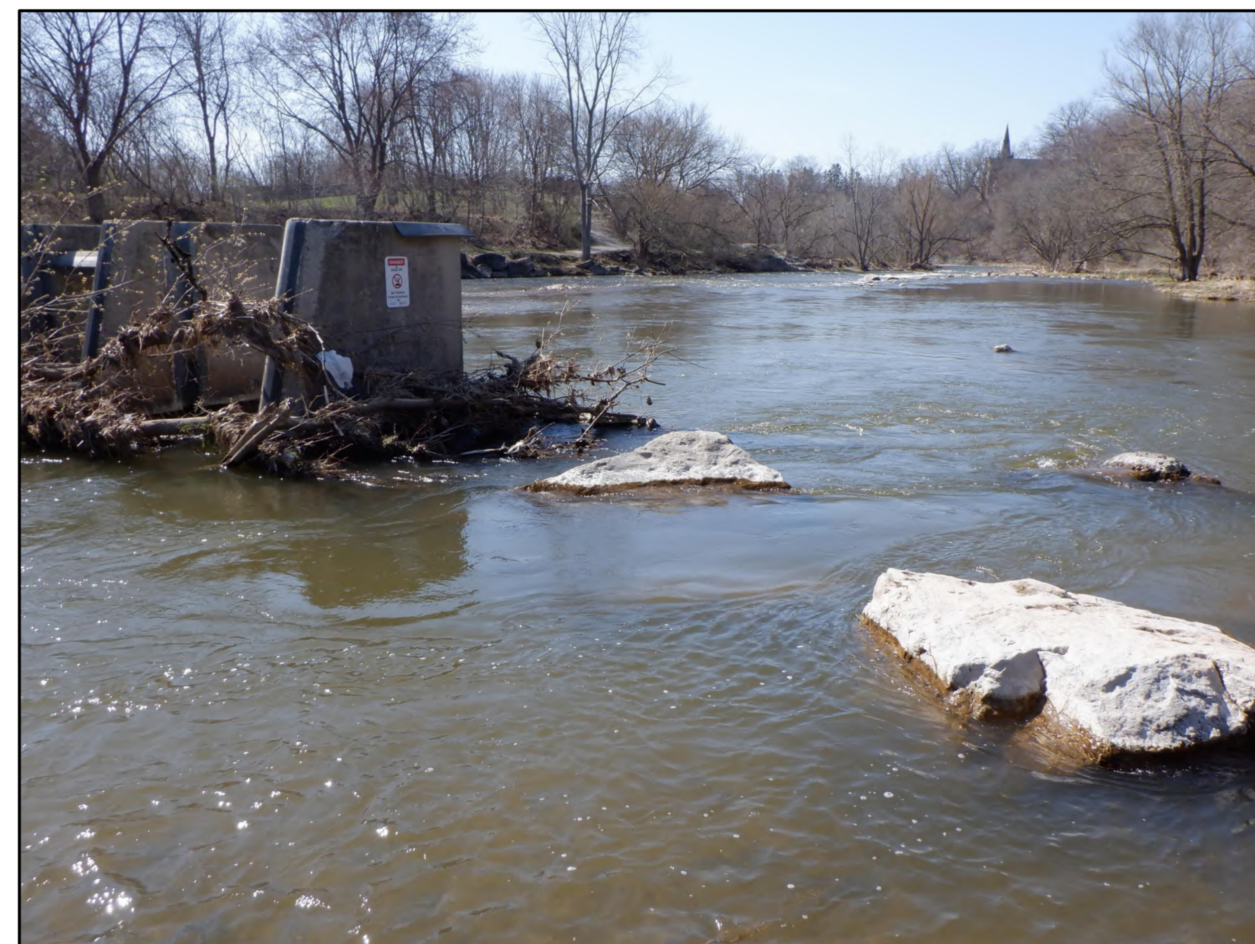
By-Passed Ice Control Structure
