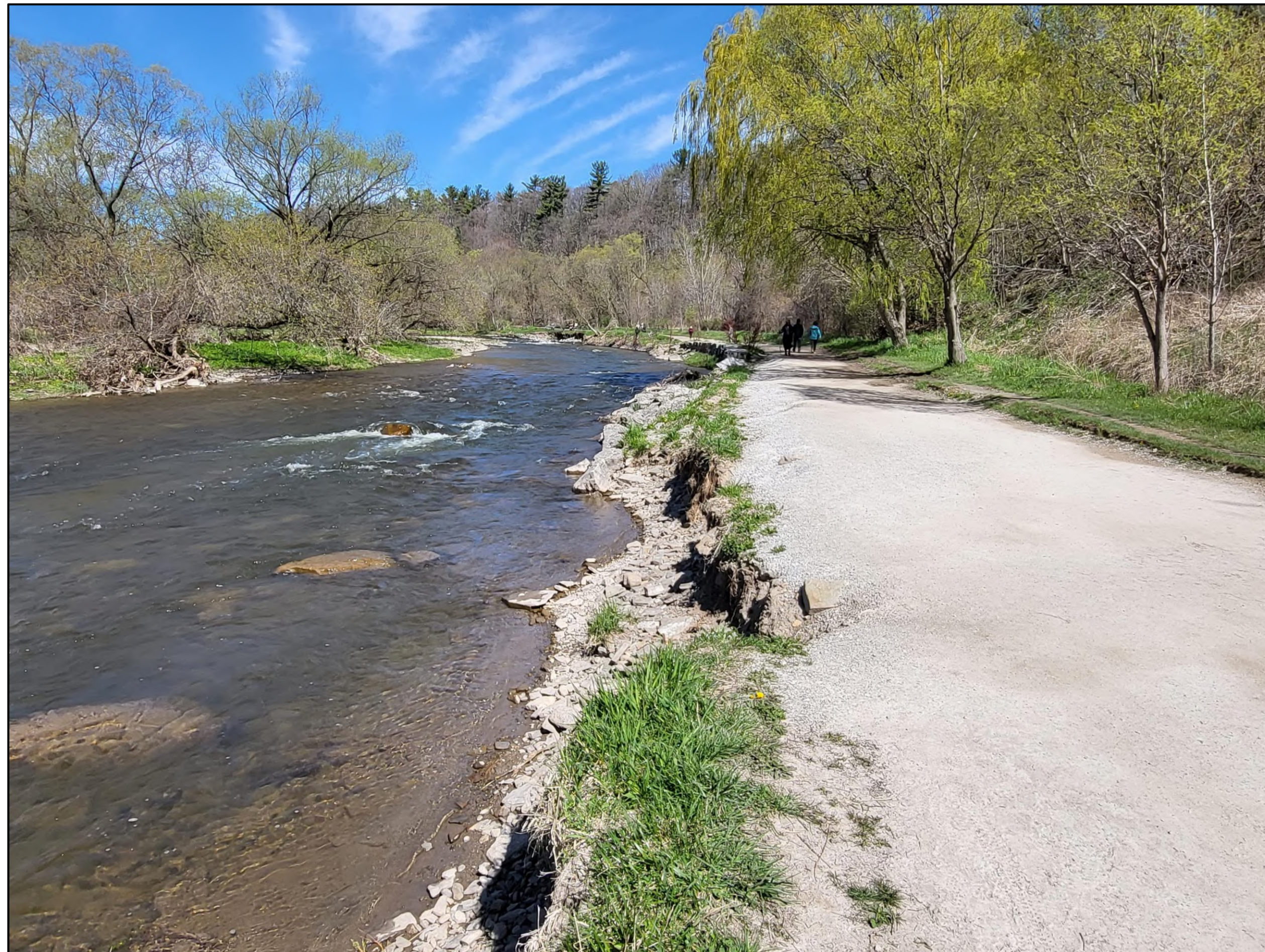
Bank Erosion Along Culham Trail
