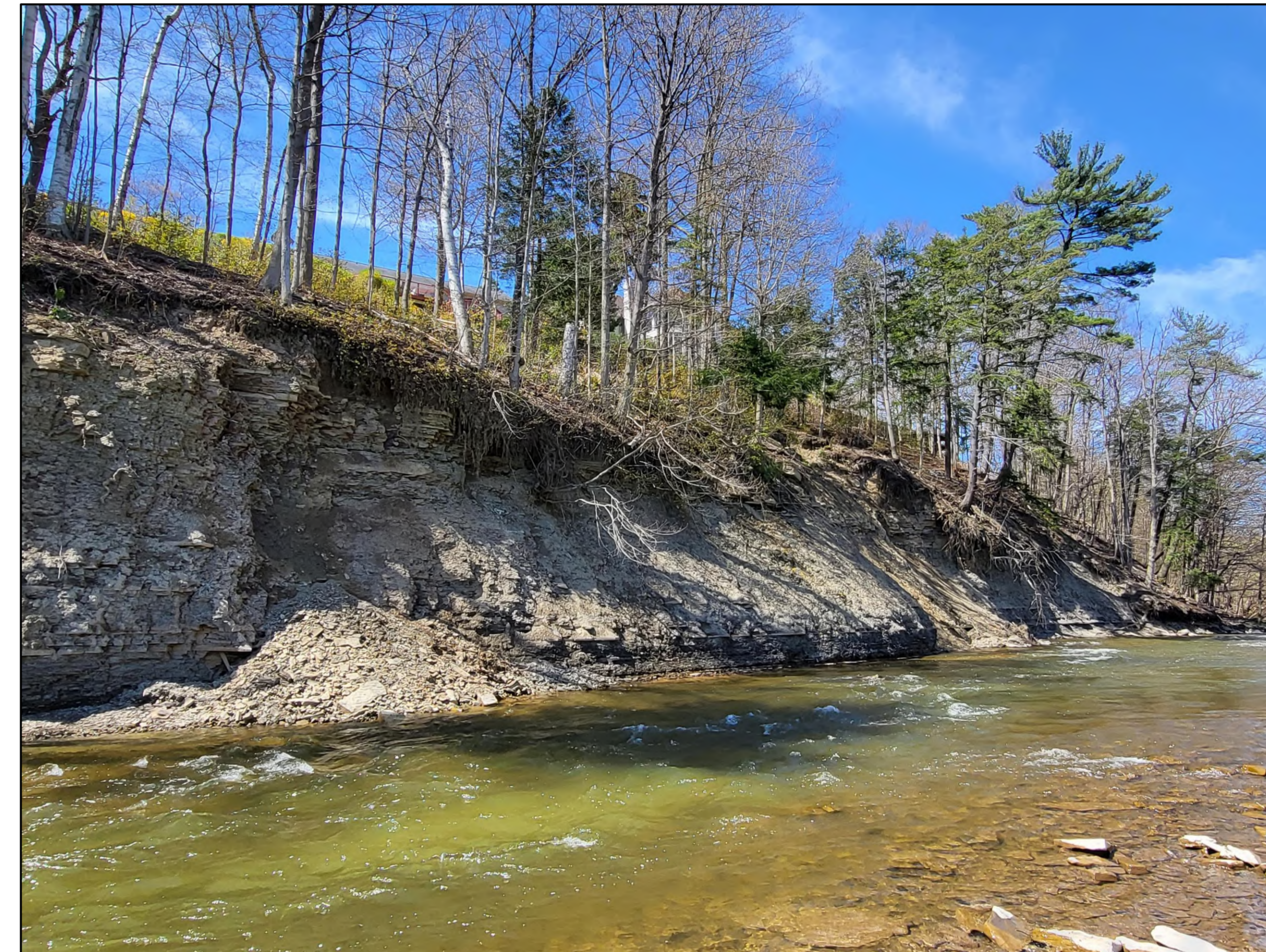
Valley Wall Erosion and Slope Instability
