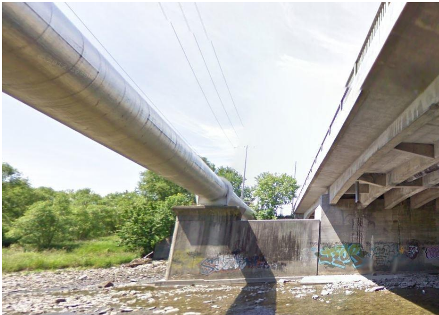
Image 19: View west across the Etobicoke Creek, Lakeshore Road to the north and large sewer pipe running east west in the ROW immediately south of the road
