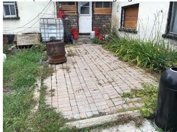
16. View of the side door and access to basement/crawl space on the south side of the house, looking north.
