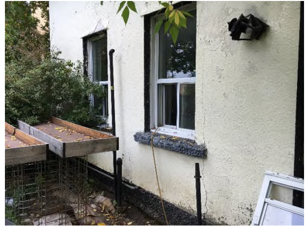
2. View of the fill and vent pipes along the west wall of the house, looking northeast.
