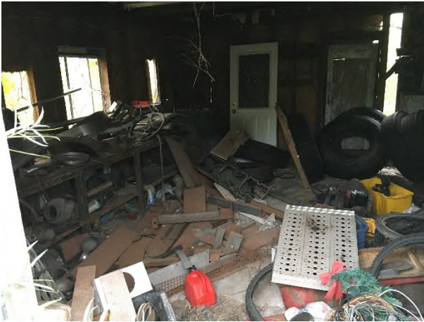
13. View of various garbage items inside the wooden shed at the southeast corner of the Site, looking south.
