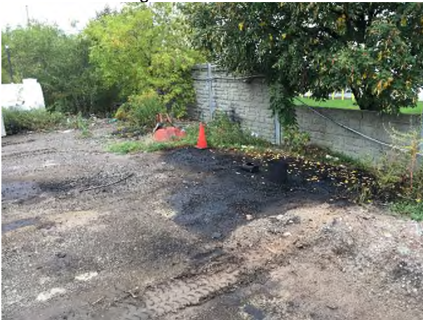
11. View of heavily stained ground west of the diesel tanks at the southeast portion of the Site, looking southeast.
