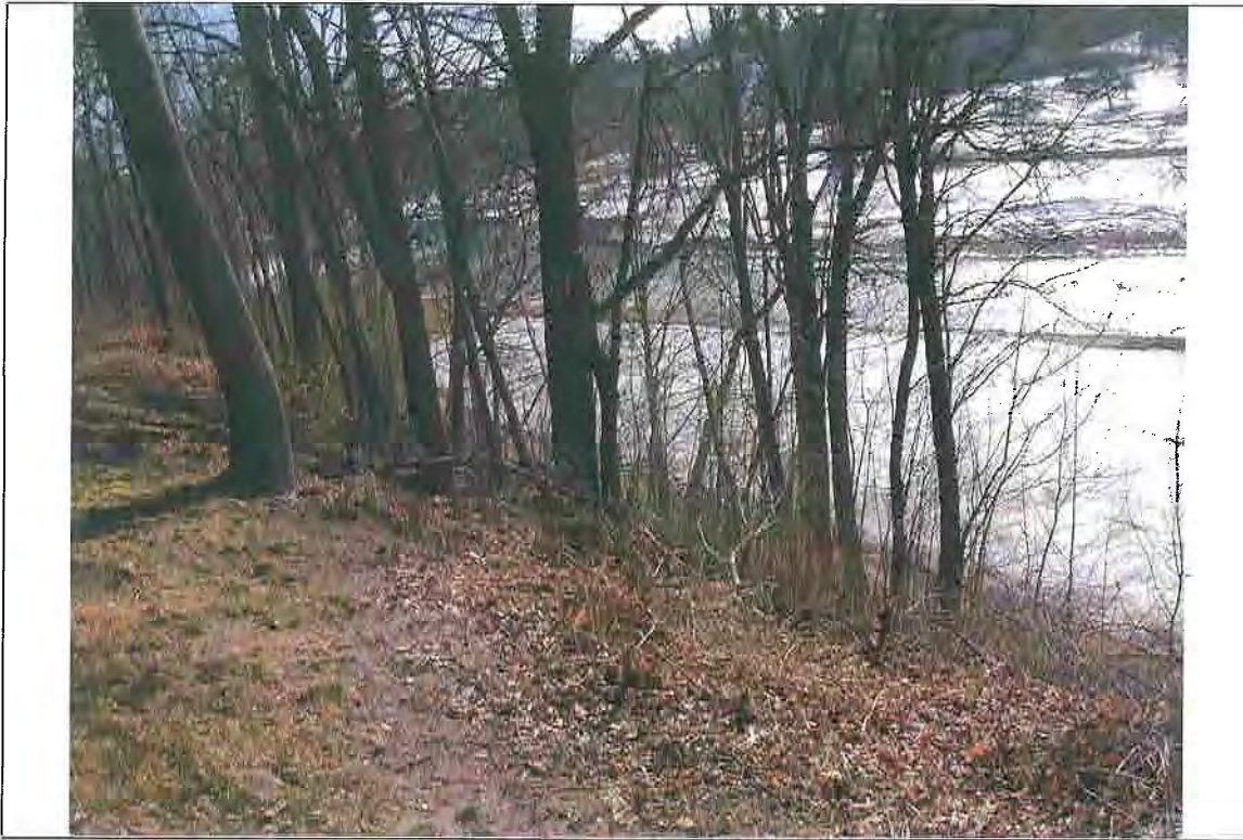
Photo No 3 – Upper Section of the Slope Cross Section
