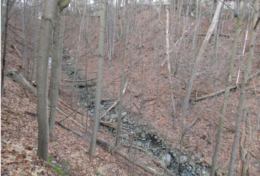
PHOTOGRAPH 11. Looking north, a view of the slope toe. A relatively shallow drainage swale is situated at the slope toe before the slope rise again on the other side of the swale.
