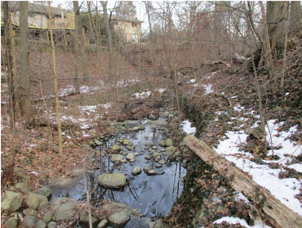
PHOTOGRAPH 19. Looking southeast, a view of the slope toe and drainage swale. The swale bank includes field stone/gabion lining.
