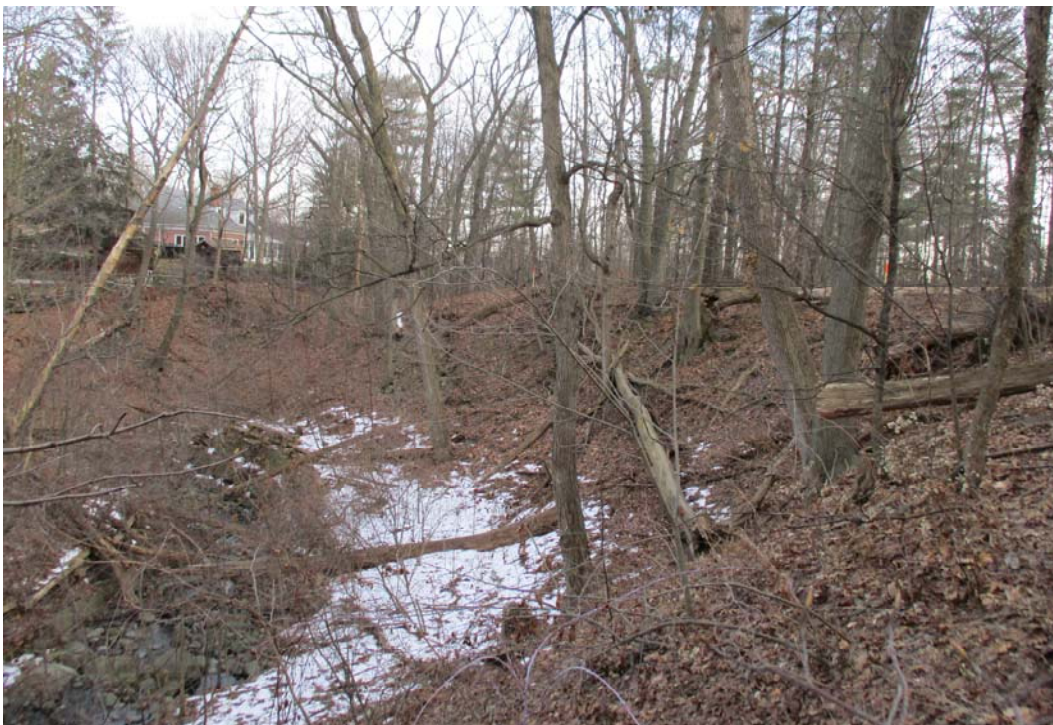
PHOTOGRAPH 18. Looking southeast, another view of the ravine slope and drainage swale. The swale bank includes field stone/gabion stone lining. No evidence of the slope toe/swale bank erosion.
