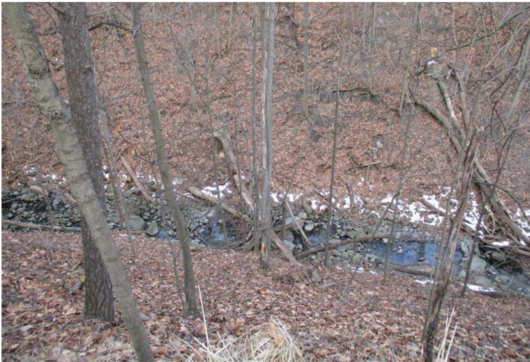
PHOTOGRAPH 14. Looking northeast, a view of the slope toe and drainage swale. The swale surface is covered with numerous field stone and cobbles. No evidence of bank erosion.
