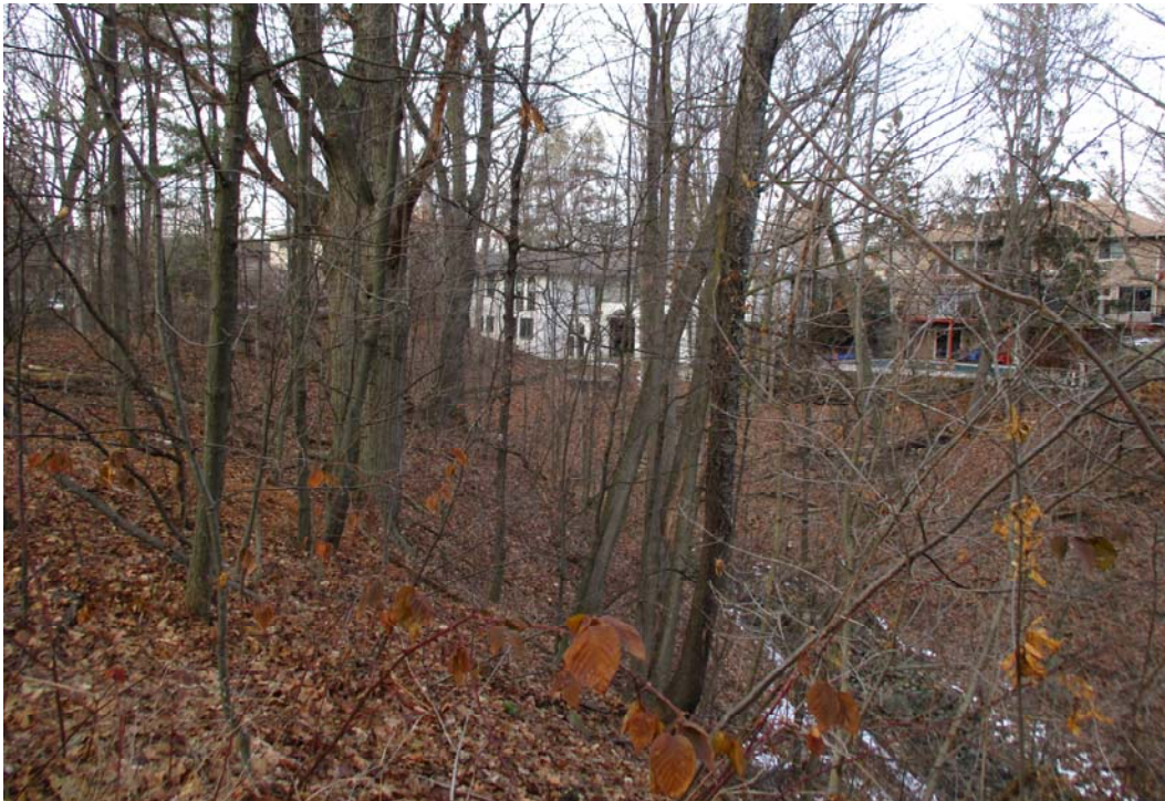
PHOTOGRAPH 17. Looking northwest, another view of the vegetated ravine slope. No conspicuous evidence of slope instability and toe erosion.
