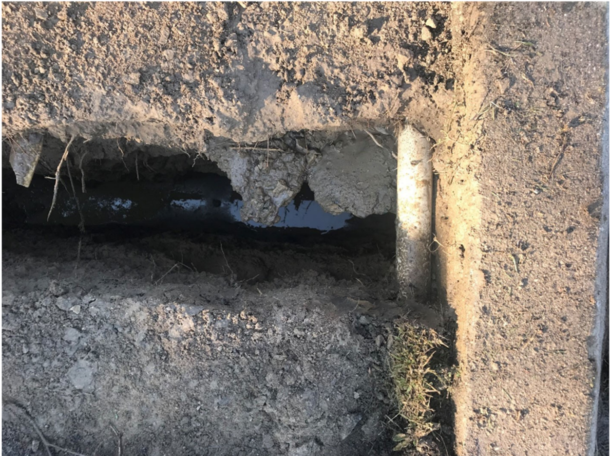
Image 1: Existing streetlight conduit behind barrier curb along Kirwin Ave. (Provided in initial report dated August 27, 2021)
