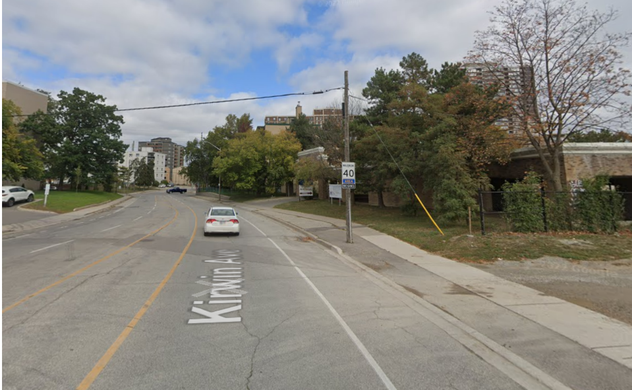
Image 2: Existing Bell pole with overhead wiring along the western property line of 3085 Hurontario St. and 3121 Hurontario St.
