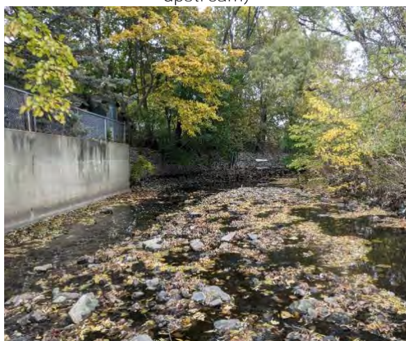
Figure 8. Channel banks transition from concrete vertical wall to Gabion baskets (looking downstream)
