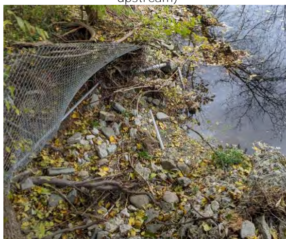
Figure 9. Failed Gabion baskets along creek bank
