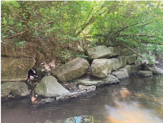
3 – Poor (Armourstone Slump)
