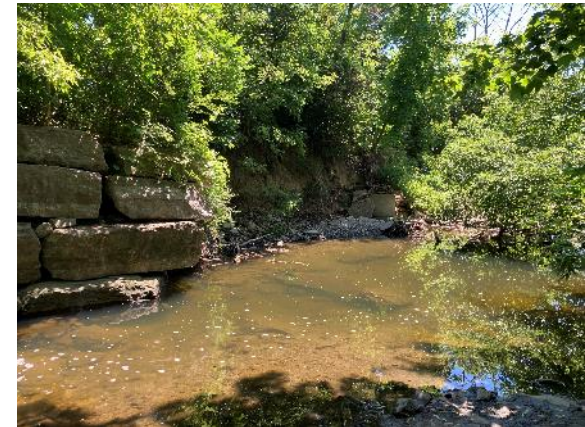
5 – Failure into Channel (Amourstone)
