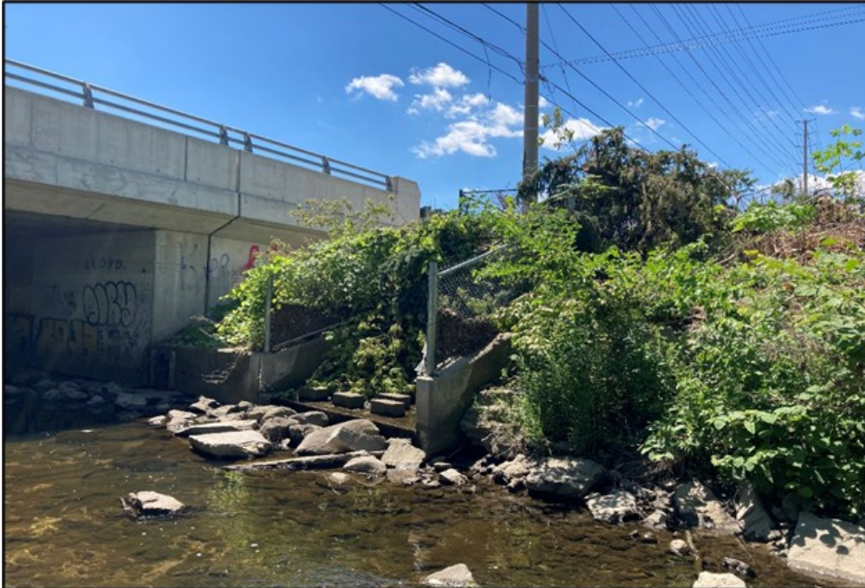
11. Reach R3 – Outfall on right bank upstream of Dundas Street Crossing; toe of bank is lined with remnants of riprap.
