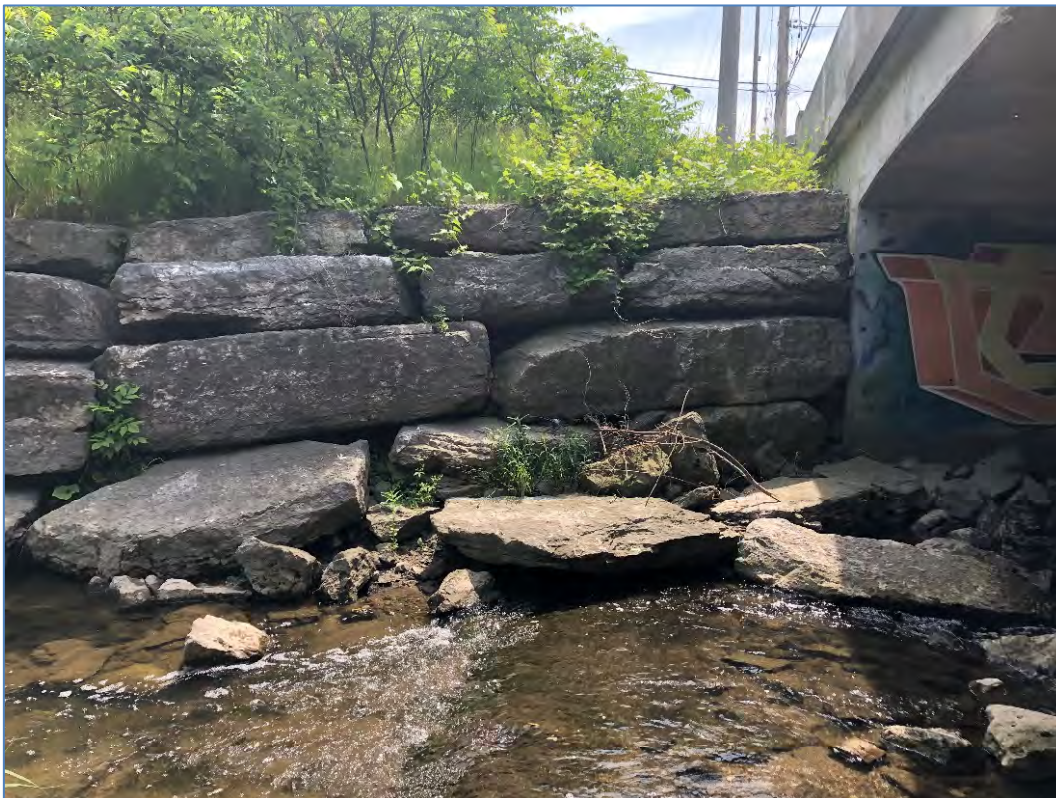
Photograph 8: R2b view of armourstone on right bank and concrete feature on bed
