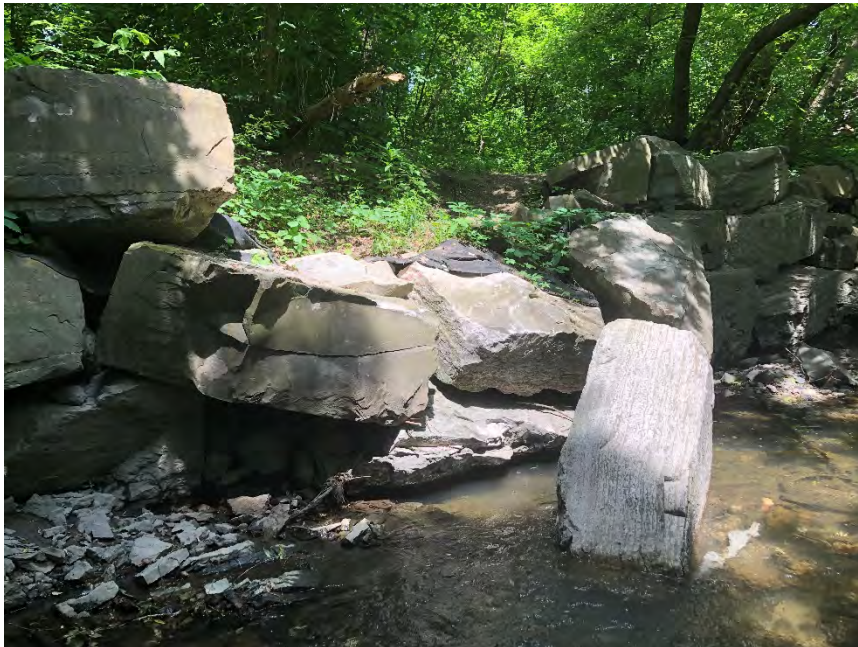
Photograph 12: R2b failed armourstone treatment
