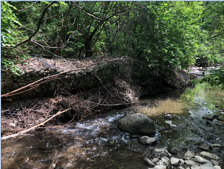
Photograph 18: R3 view downstream of failed gabion baskets on left bank
