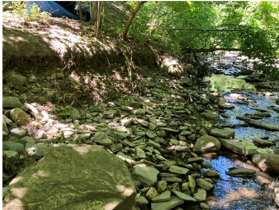
3 – Moderate Bank Erosion
