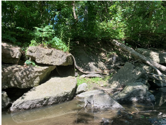
4 – Failure on Bank (Armourstone)
