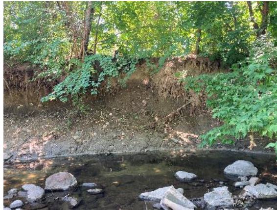
4 – Major Bank Erosion
