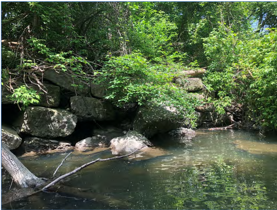
Photograph 10: R2b view of failed armourstone bank treatment on right bank
