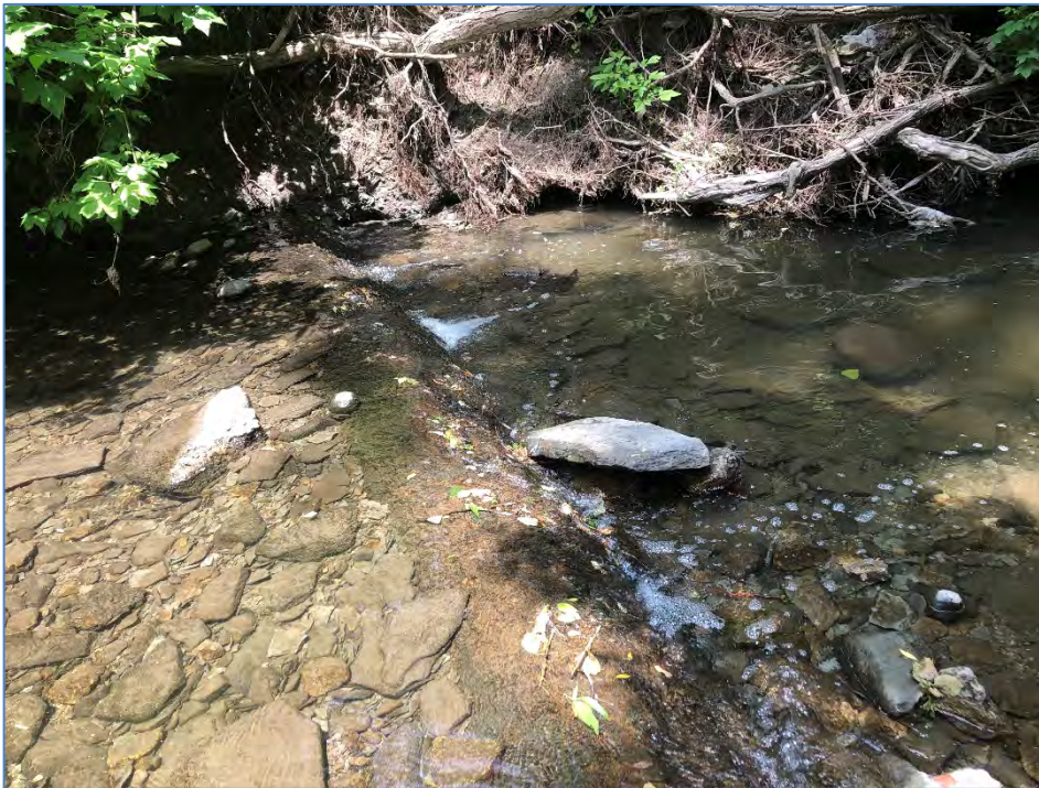
Photograph 15: R3 potential exposed pipe on bed of channel
