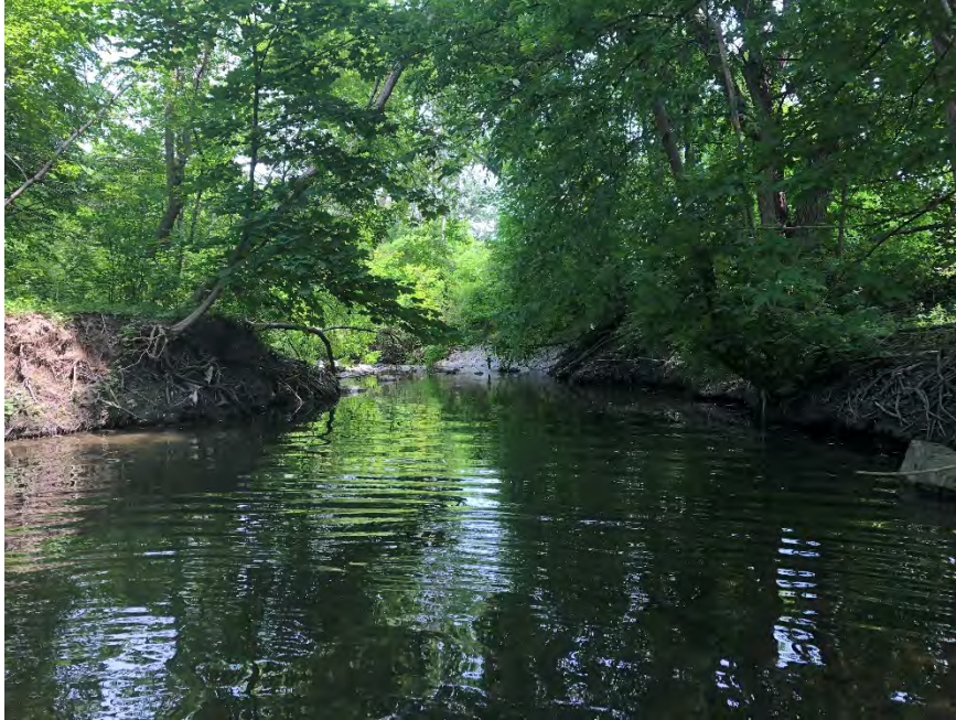
Photograph 12: R3 view downstream of widened section with bank erosion on right bank
