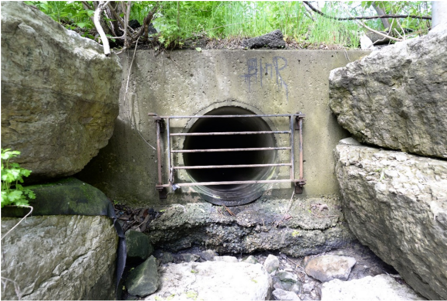
Photograph 4: Looking north at stormwater outfall structure located approximately 7 m downstream of Dixie Road Bridge.
