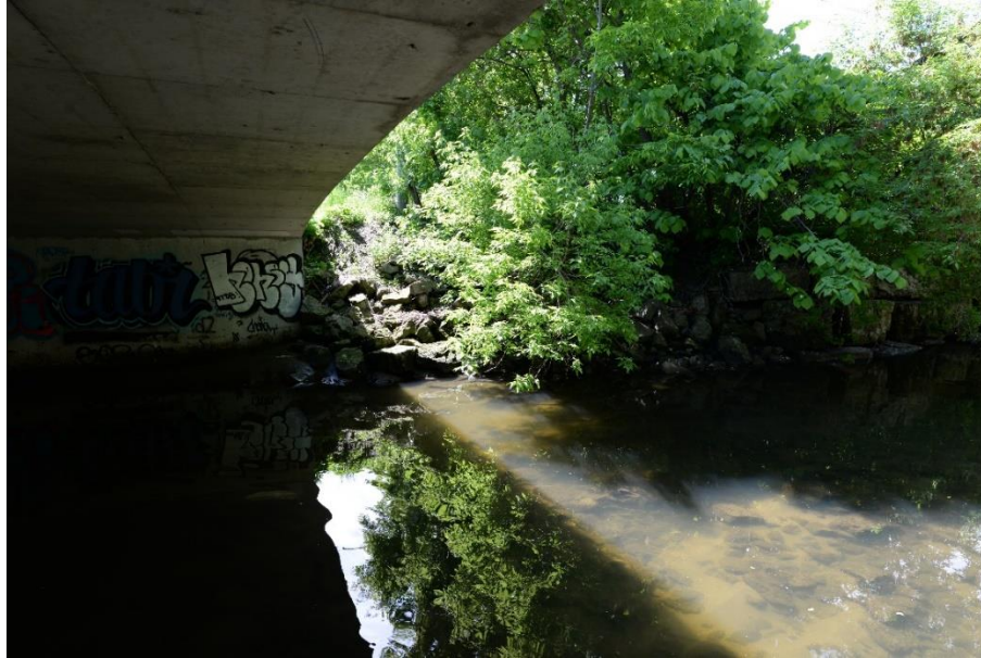
Photog 7: Looking south from west side of Dixie Road bridge. [taken June 2019]
