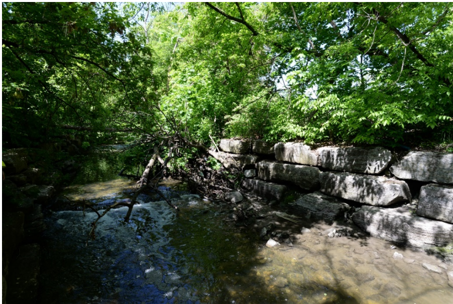
Photograph 10: Looking upstream at a fallen tree located approximately 50 m west of Dixie Dundas Bridge.
