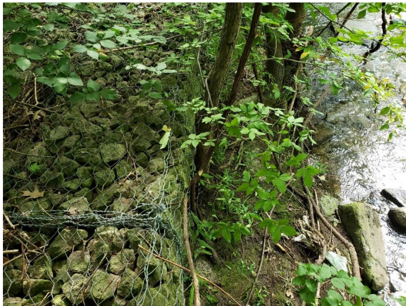
Photo 20: Looking at gabion baskets along east bank at Willowcreek Park. [taken June 2019]
