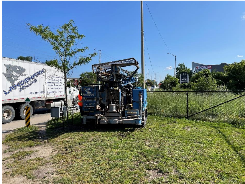
Photo 3. Looking east along Dundas Street East towards drill rig setting up at DUN-01. [taken August 2021]
