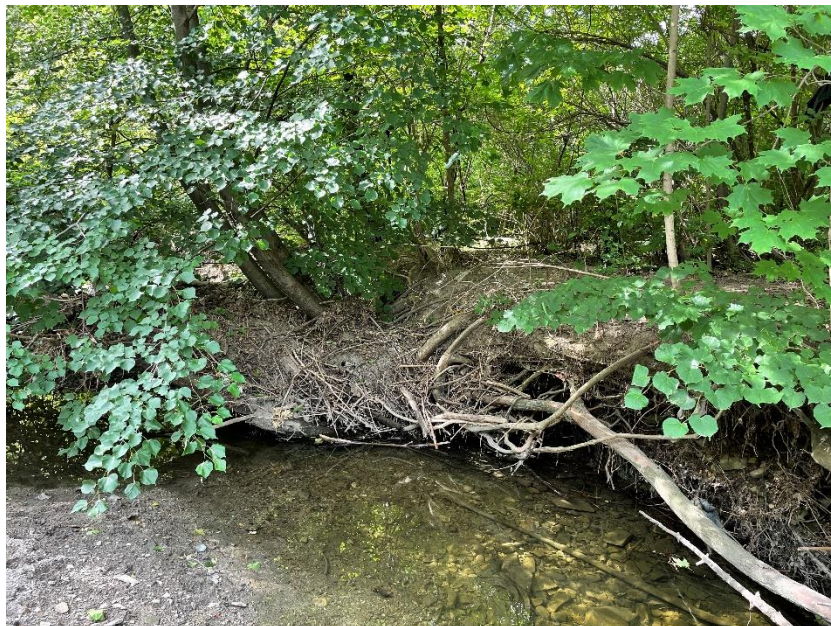
Photo 29: Looking west towards undermining along west bank 300 m downstream from Dundas Street East bridge. [taken June 2021]
