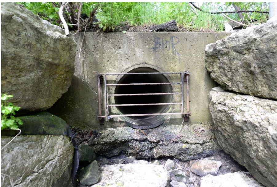
Photo 4: Looking north at stormwater outfall structure located approximately 7 m downstream of Dixie Road bridge. [taken June 2019]
