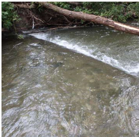
FIGURE 3 Exposed 450 mm Sewer in Little Etobicoke Creek
