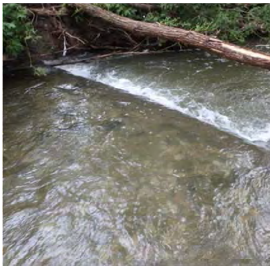
FIGURE 3 Exposed 450 mm Sewer in Little Etobicoke Creek
