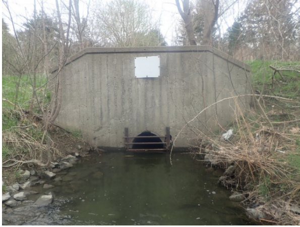
PHOTOGRAPH 9 A 750 mm diameter Stormwater Outfall Enters the Channel on the North Bank of Cooksville Creek Upstream of the Mississauga Valley Boulevard Crossing; the Concrete Outfall was Grated and had a Concrete Headwall Structure
