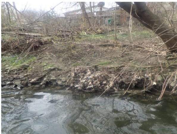
PHOTOGRAPH 3 Emptied Gabion Cage Remains Intact with Channel Bank; Gabion Stone has been Disbursed from the Erosion Protection
