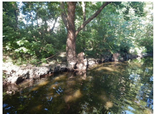
PHOTOGRAPH 4 Degraded Gabion Cage; Slumping and Deformation of the Erosion Control Measure, Some Gabion Stone has Washed into Channel
