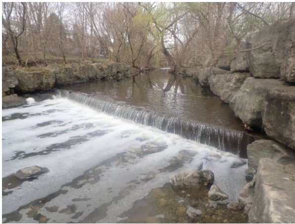
PHOTOGRAPH 5 Concrete Sanitary Sewer Encasement at Sewer Crossing 0+240 ; Sanitary Sewer Encasement Creates a Maximum Drop in Bed Elevation of 0.64 m
