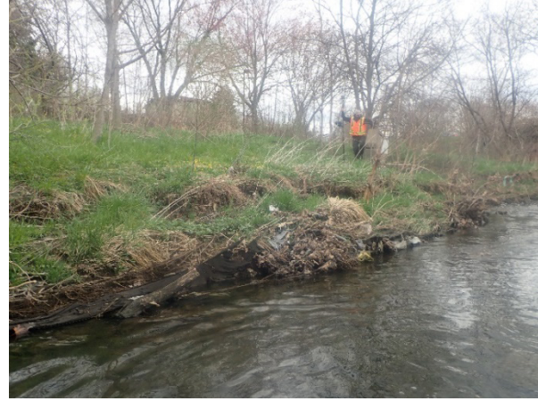
PHOTOGRAPH 12 Slumping Bank Material Directly Upstream of the 750 mm Concrete Stormwater Outfall (North Bank); Located Near Upstream Limit of Study Area
