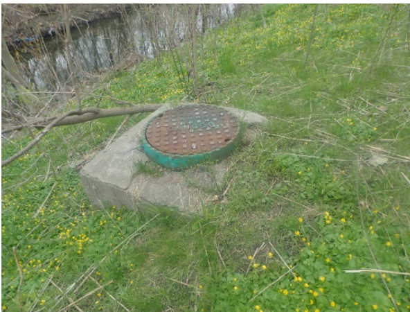
PHOTOGRAPH 15 Manhole within the Cooksville Creek Corridor Associated with a Sanitary Sewer Crossing
