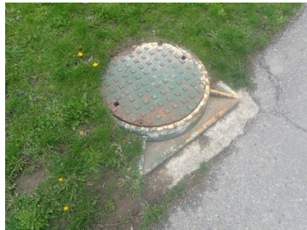
PHOTOGRAPH 16 Manholes Exist Along the Pedestrian Pathway and are Generally Associated with the Sanitary Sewer which Runs Parallel to Cooksville Creek
