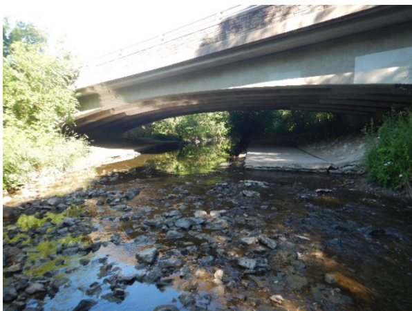
PHOTOGRAPH 13 Scour of Channel Banks has Occurred on the Upstream South Side of the Bridge Inlet
