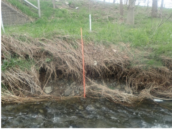
PHOTOGRAPH 11 Vertical Eroded Bank with Exposed Roots and Gravel and Sand Material within the Bank; Located Directly Downstream of Mississauga Valley Boulevard (North Bank)
