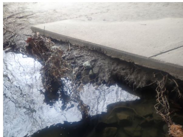
PHOTOGRAPH 14 Corrosion of Gabions Underneath the Concrete Slabs
