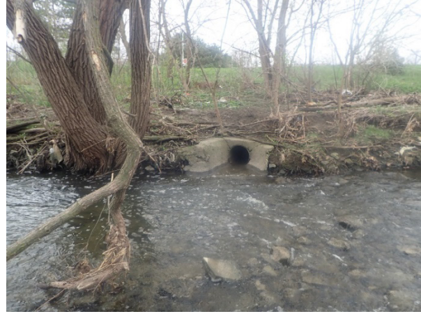
PHOTOGRAPH 10 A 400 mm diameter Storm Outfall on the South Bank of Cooksville Creek Upstream of the Mississauga Valley Boulevard Crossing
