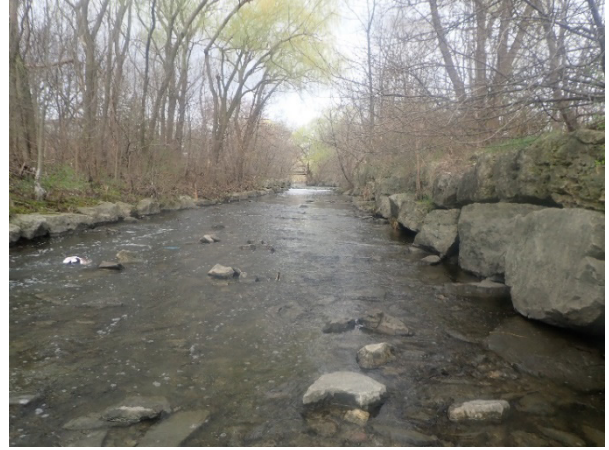
PHOTOGRAPH 2 Upstream View of Channel Cross-section, North Bank (right) Protected by Three-tiered Armourstone Wall, South Bank (left) Protected by Single-tier Armourstone Wall
