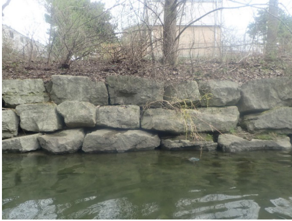
PHOTOGRAPH 1 Three-tier Armourstone Protection on the North Bank of Cooksville Creek, Armourstone Intact, Vegetation Establishment on Top of Armourstone Wall
