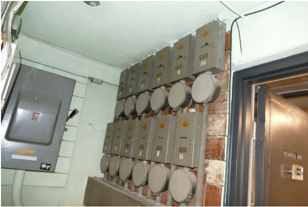
P13 - Interior of the Mechanical Room
