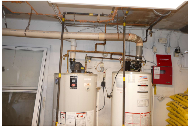
P14 - Hot Water Boilers Within the Mechanical Room
