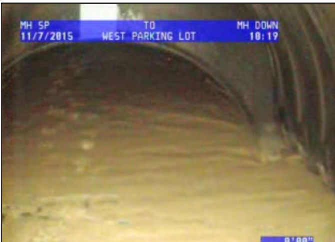
SEPARATOR ROW: Separator Row prior to cleaning
