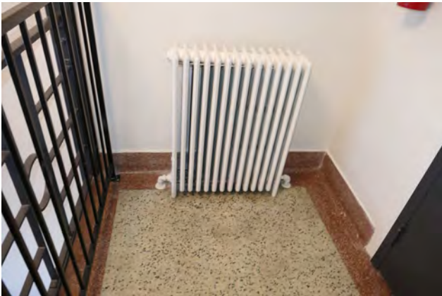
P10 - Typical Hot Water Radiator Observed Within the Stairwells
