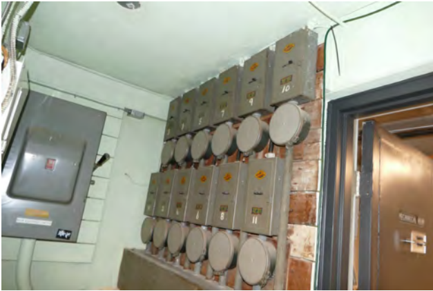
P13 - Interior of the Mechanical Room
