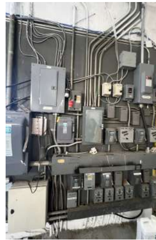
Photo 10: View of electrical panels inside the sprinkler room in Building A (1970 Fowler Drive), facing north
