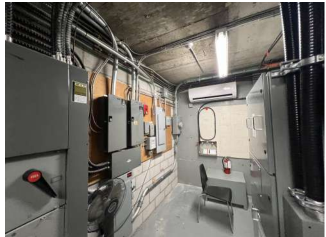
Photo 22: View of the electrical room in the basement of Building B (1980 Fowler Drive), facing east.
