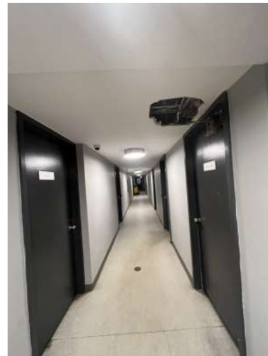
Photo 4: View of the basement hallway and the leakage in the ceiling from water leak in Building A (1970 Fowler Drive), facing north.
