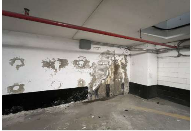
Photo 8: View of the water leakage in the west corner of underground parking garage in Building A (1970 Fowler Drive), facing southwest.
