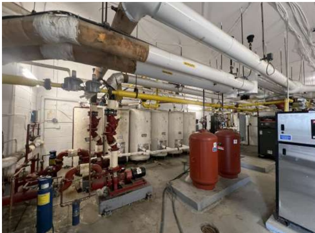
Photo 9: View of fire sprinkler system on the roof of Building A (1970 Fowler Drive), facing southwest.
