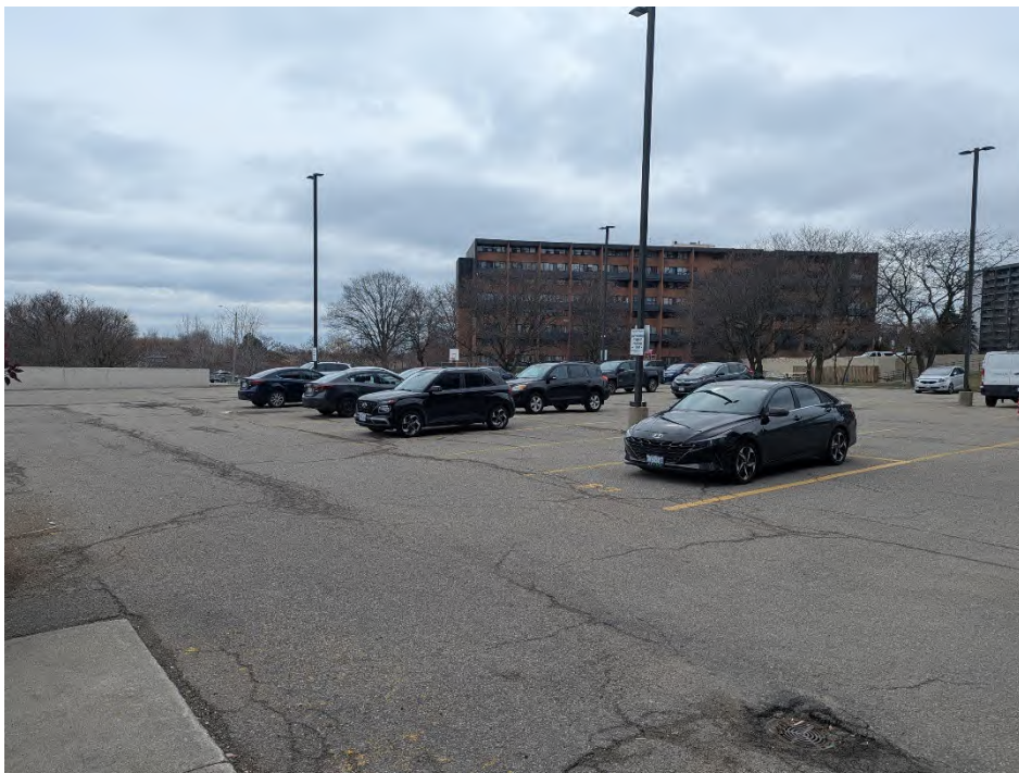
Image 16: View southeast across the 1980 Fowler surface parking lot (built over underground garage).
