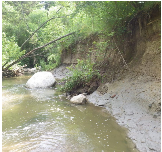
Figure 4.7. Sawmill Creek is in need for rehabilitation, as erosion impacts the channel banks and woody debris, posing significant risks to the adjacent trail, sanitary sewer infrastructure and the environment. (c. City of Mississauga)
