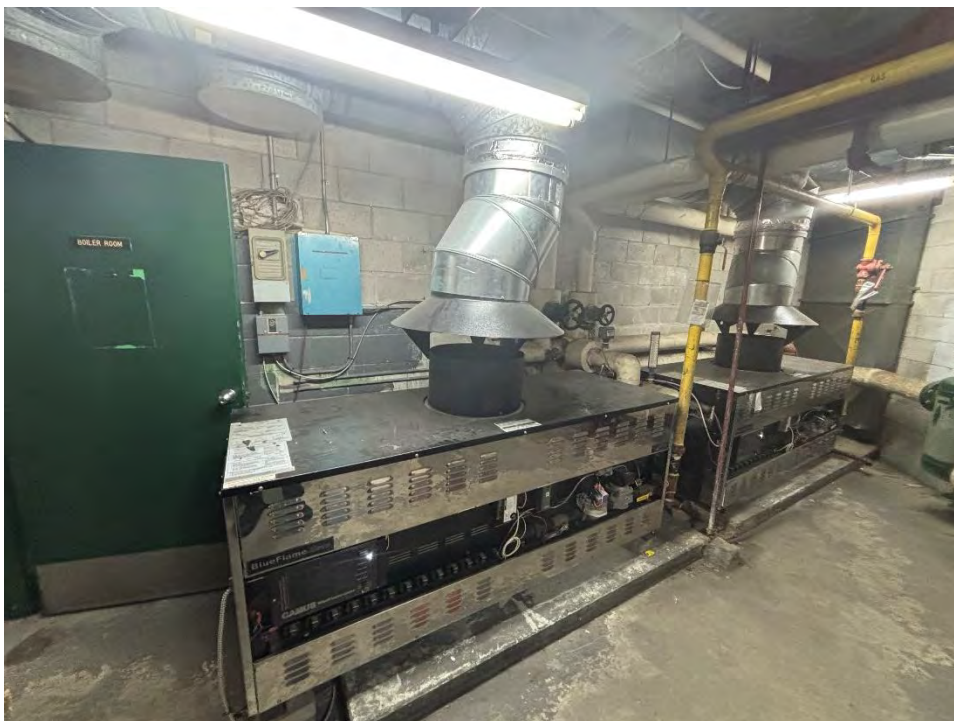
Photograph 24: View of the boiler room of Building B at the Property.
