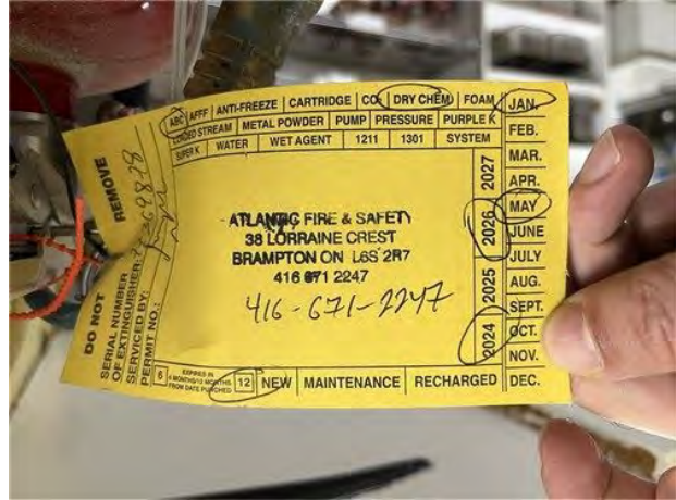
Fire Extinguisher Tag
