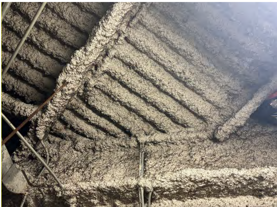
Photograph 20: View of potential friable asbestos-containing sprayed fireproofing located on the ceiling deck of Building B at the Property.
