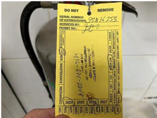
Type K Extinguisher Tag
