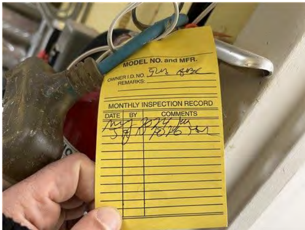
Fire Extinguisher Tag
