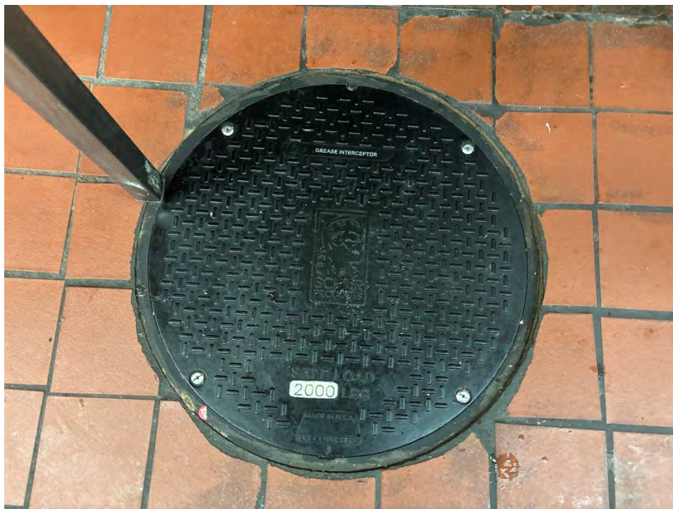
Photograph 26: View of the grease interceptor located in Unit 106 (Swiss Chalet) in Building A at the Property.
