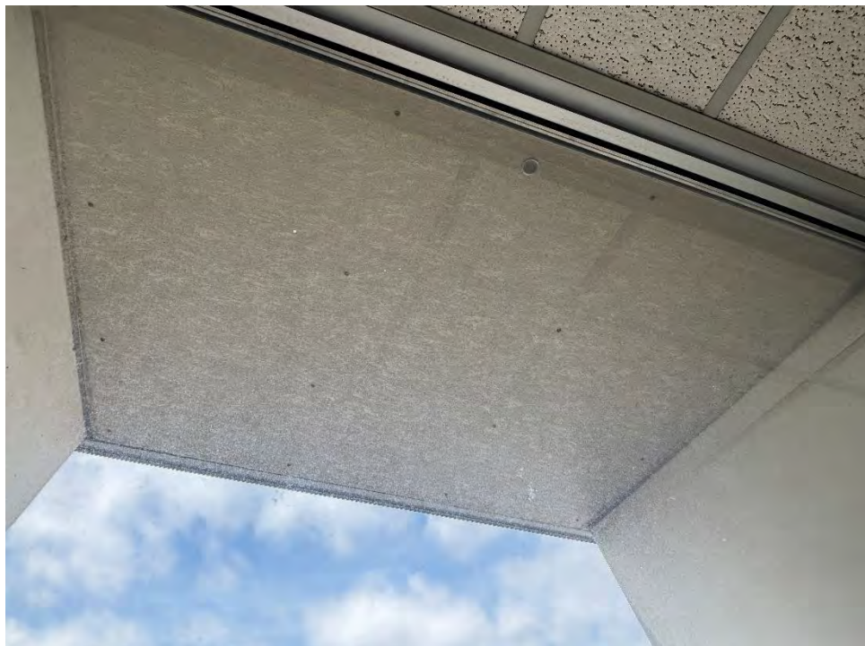
Photograph 19: View of potential non-friable asbestos-containing Transite cement panels on the exterior canopies of Building B at the Property.
