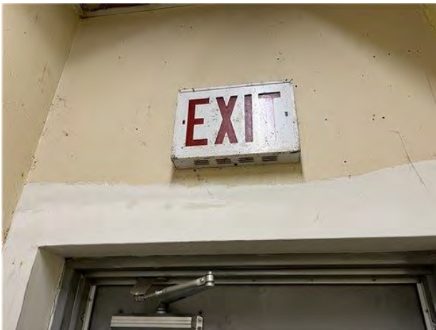
Emergency Exit Signage
