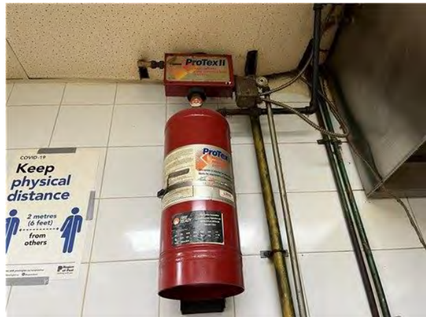
Fixed Fire Suppression System
