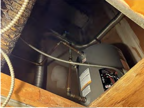
Hot Water Tank
