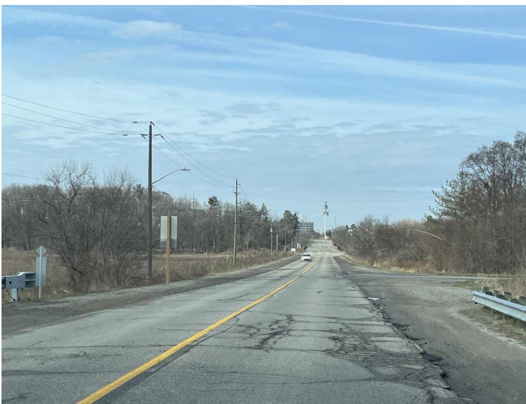
Road rehabilitation needed on Old Derry Rd (Gazette Gate to Lessard Lane)
