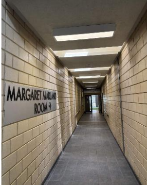
LED Interior Lighting
