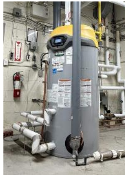
High Efficiency Water Heater
