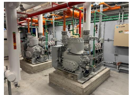
Ice Plant Compressors
