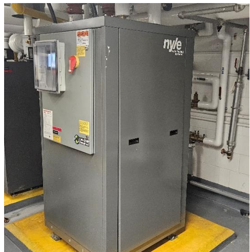
Heat Pump Water Heater
