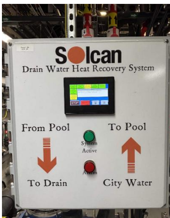
Pool Drain Heat Recovery
