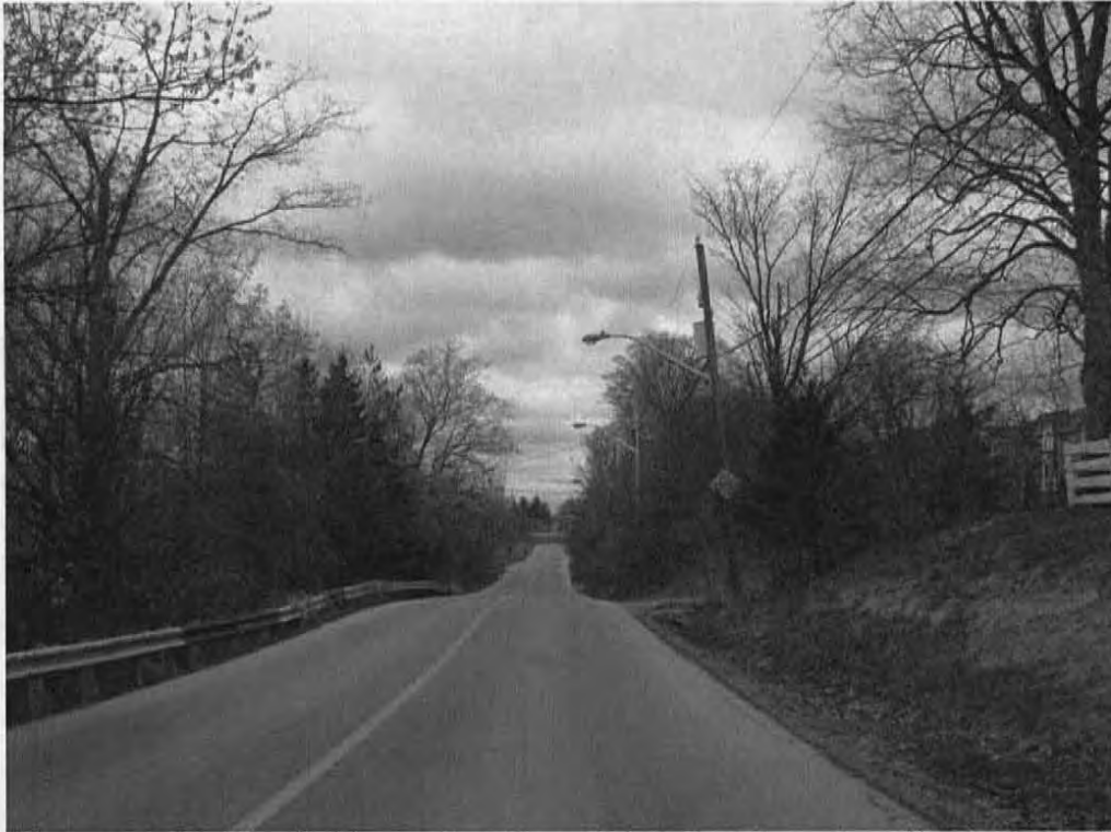
Photograph #3 - View looking north on Second Line of existing poles with primary conductors (8.32 kV)
