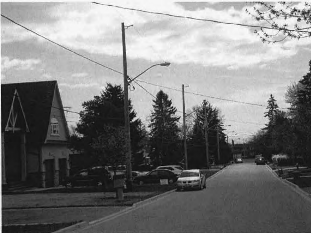
Photograph #4 – Typical 45 foot wood pole installation with primary conductor (16 kV)
