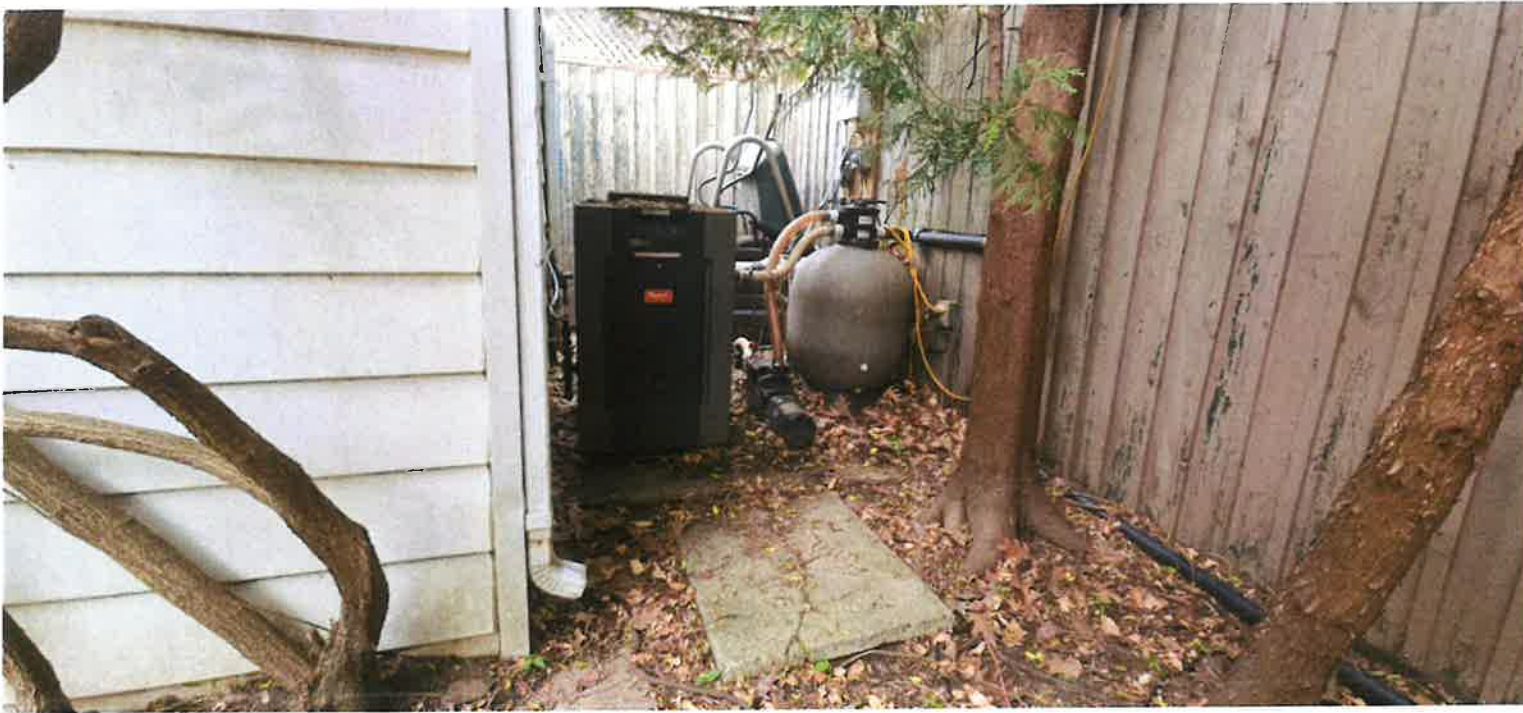
General view of the filter and pump for the pool system located east of the second shed (looking northeast)
