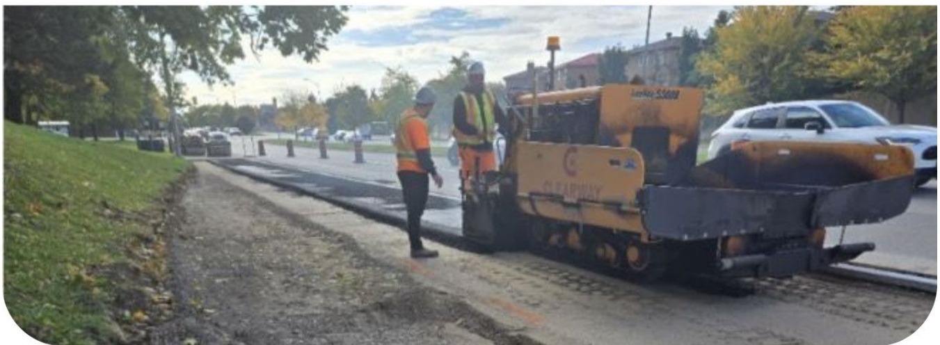
Figure 2: Construction for the new bus loop at Central Parkway Transitway Station commences.
